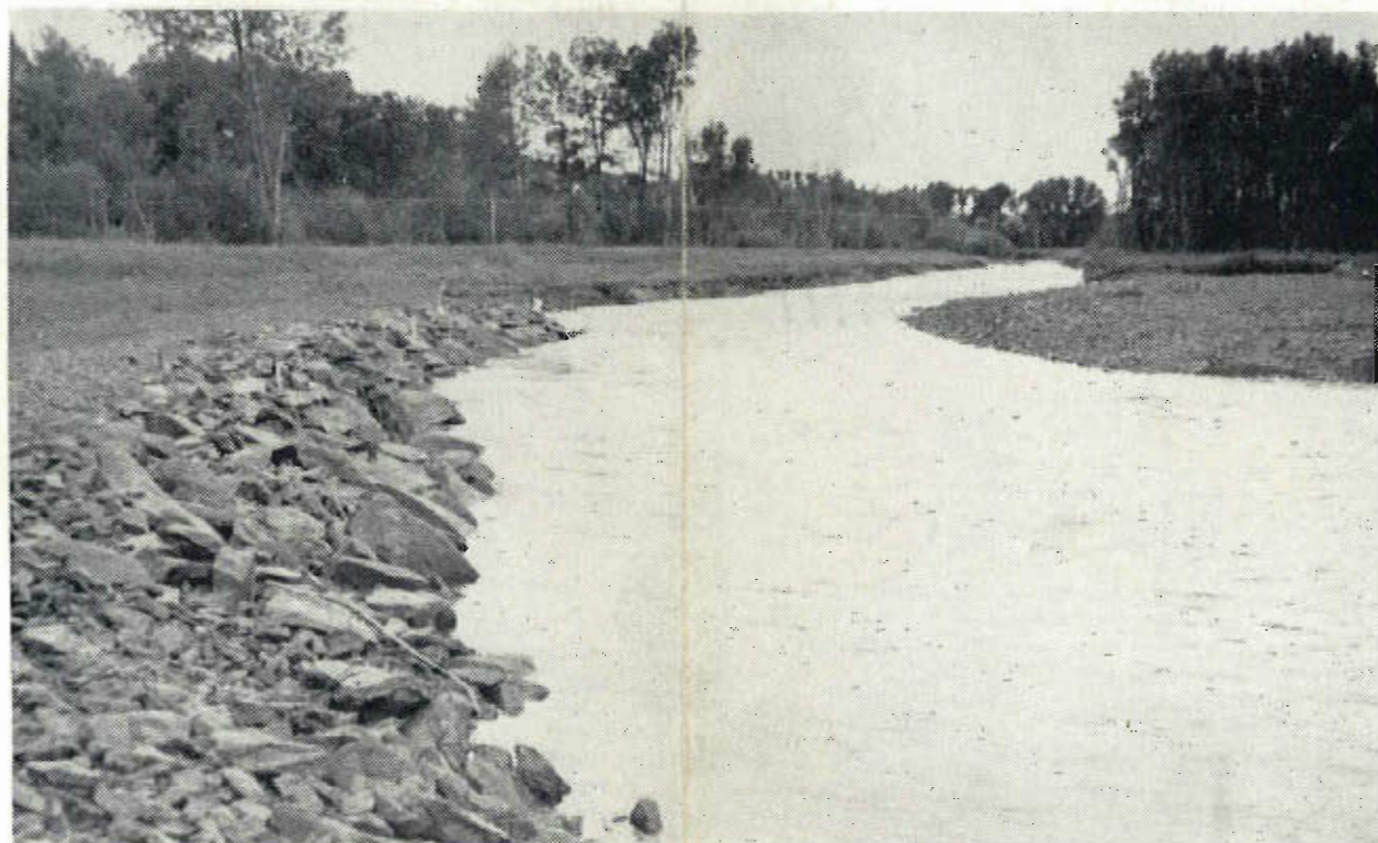
Flood control dike on the Shields river at the Keyes Bros. ranch on the west side of U. S. Highway 89 four miles south of Clyde Park, Mont. This dike was constructed by the Corps of Army Engineers in cooperation with Shields Valley Soil Conservation District in 1950.
