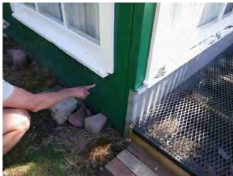
Flood Water Line, Per Owner
